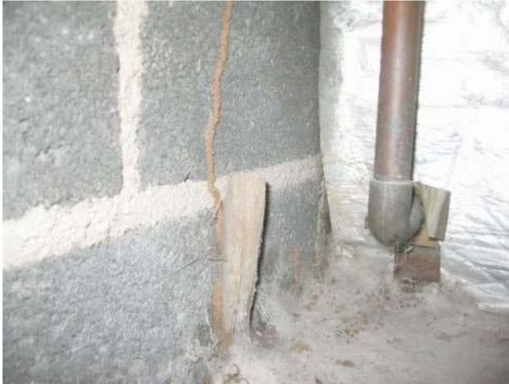
Figure 27. Termite mud tube (Courtesy of Ben Gromicko)
