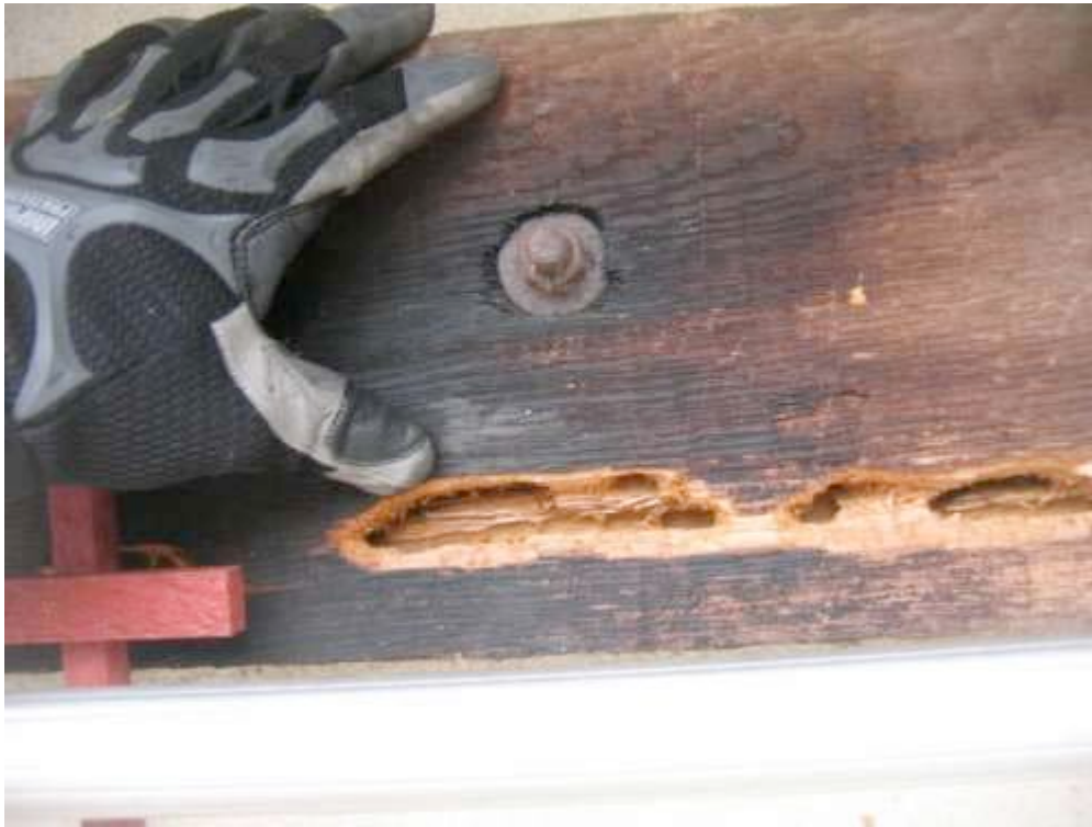
Figure 87. Carpenter bee damage (Courtesy of Ben Gromicko)
