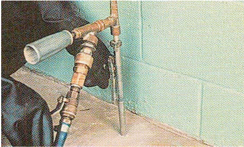
Figure 70. A slab injector is used to inject termiticide under pressure into an area beneath a slab.
