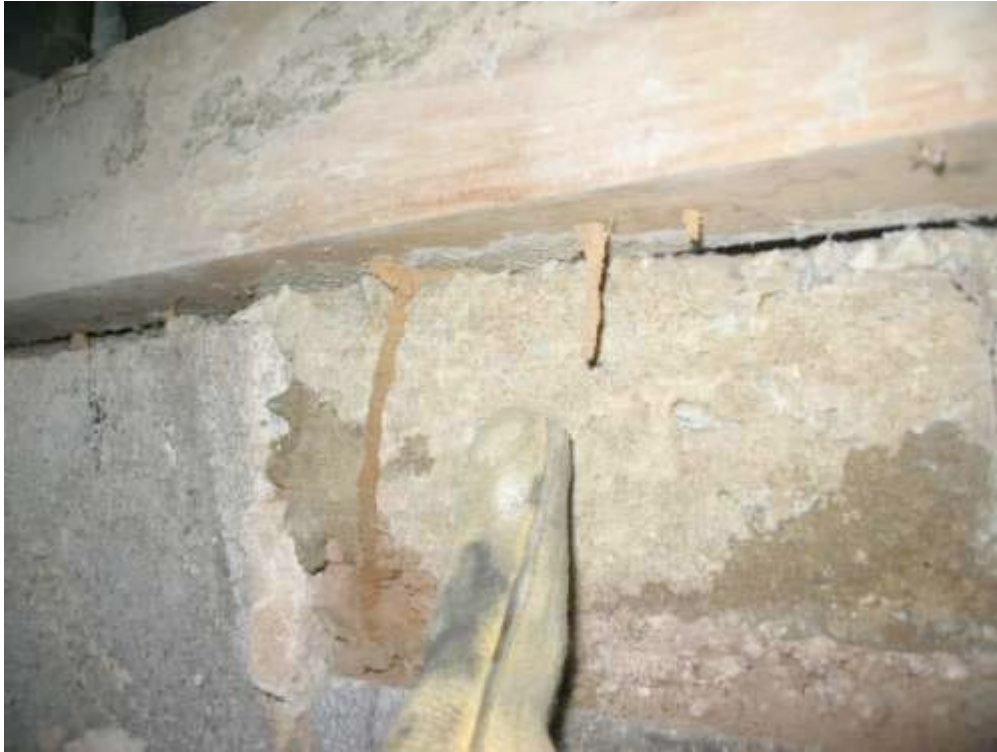
Figure 25. Termite mud tube (Courtesy of Ben Gromicko)
