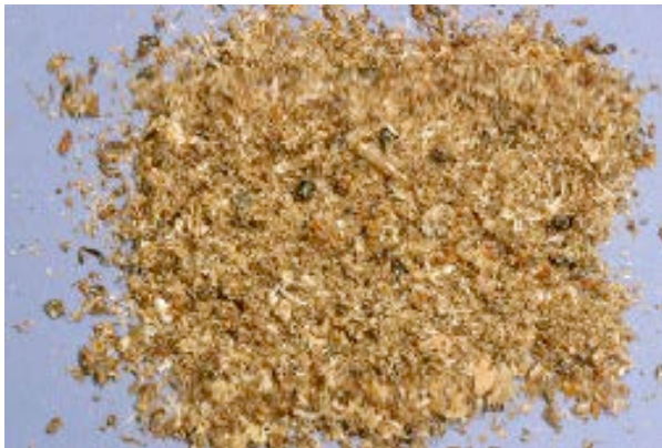
Figure 85. Carpenter ant sawdust pile
