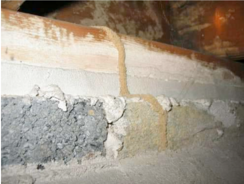
Figure 32. Termite tube on sill plate (Courtesy of Ben Gromicko)
