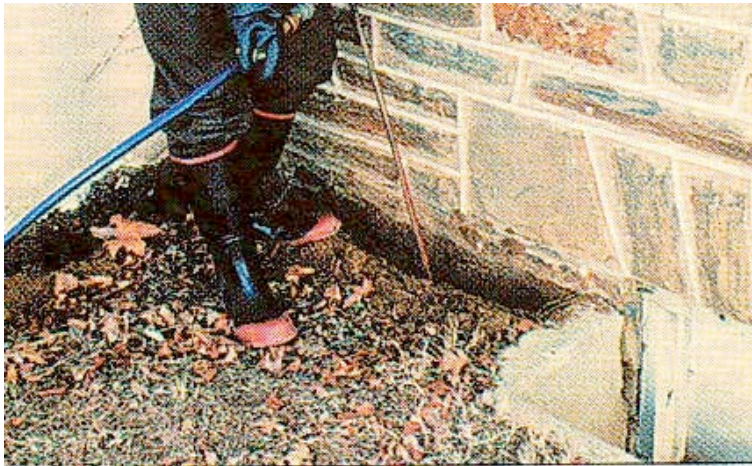
Figure 42. A typical basement treatment will also include trenching and rodding the outside perimeter of the foundation.
