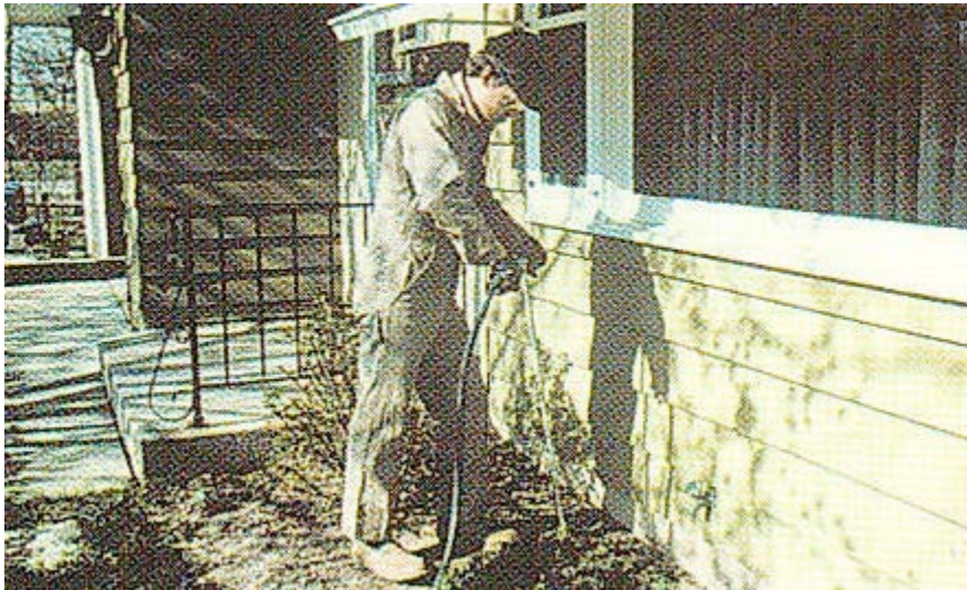
Figure 69. Pest management professional applying termiticide to the soil by long rodding the exterior of a house
