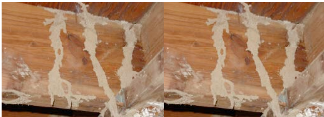
Figure 30. Termite shelter tube
