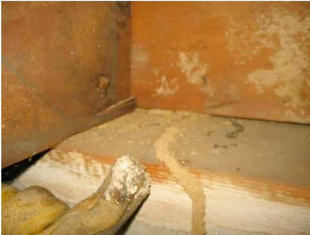
Figure 33. Termite tube on sill plate (Courtesy of Ben Gromicko)
