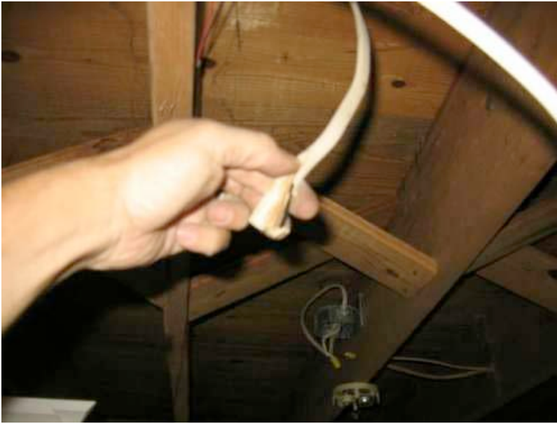
Disconnected electrical wire hanging from the basement ceiling. Deficient.
