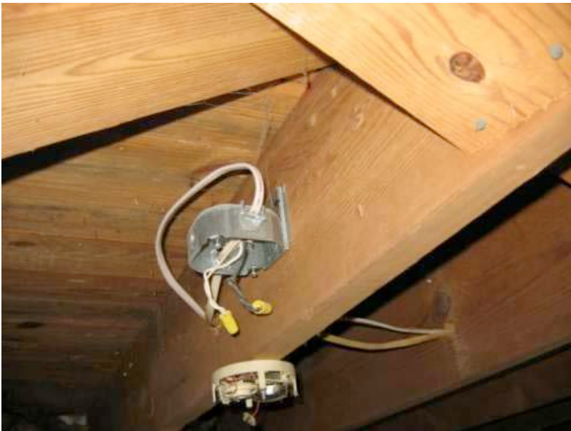
Unenclosed electrical junction box in the basement ceiling. Deficient.
