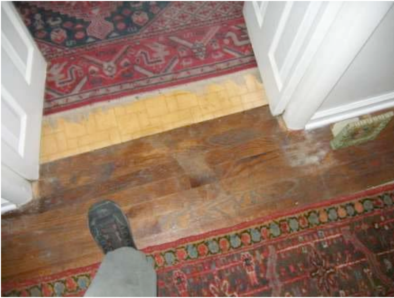
Sloping floor at the doorway between the living space and the kitchen.
