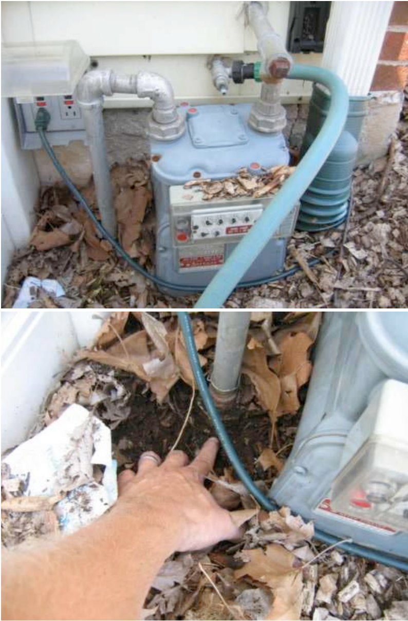
The main shut-off valve at the gas meter is buried under dirt. Deficient.
