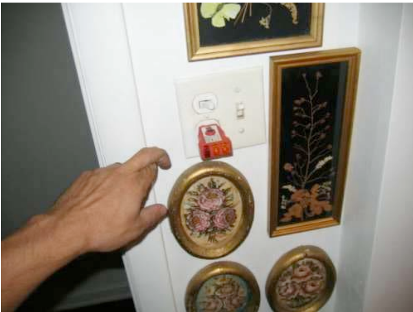
Missing GFCI protection in all of the bathrooms. Deficient.
