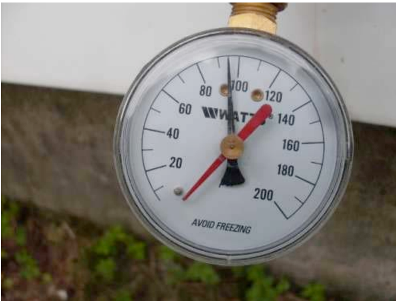
Pressure was over 80 psi, and it is considered Deficient. A pressure reducing valve (or regulator) was not found. Recommend having a plumber determine if pressure regulator is present and adjust pressure as needed. Note: No comment on pressure reducing valve is required unless the pressure is over 80. If pressure is over 80, it is automatically Deficient, and, therefore, defer inspection for the regulator to the plumber. Photo: Marcel R. Cyr. Comment John Cahill.
