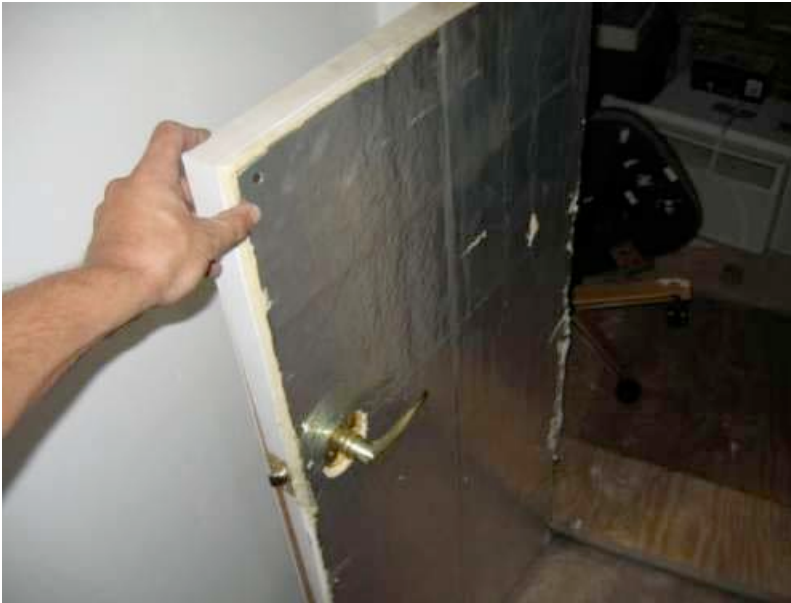
The access door to the attic space is inadequately insulated and not sealed properly. Deficient.
