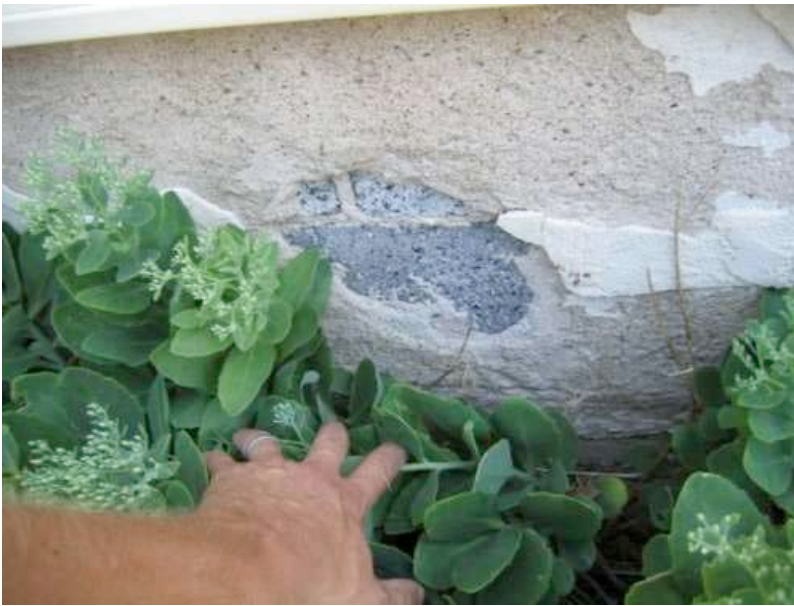
Cracking of the concrete exterior surface, located at the top of the foundation wall.
