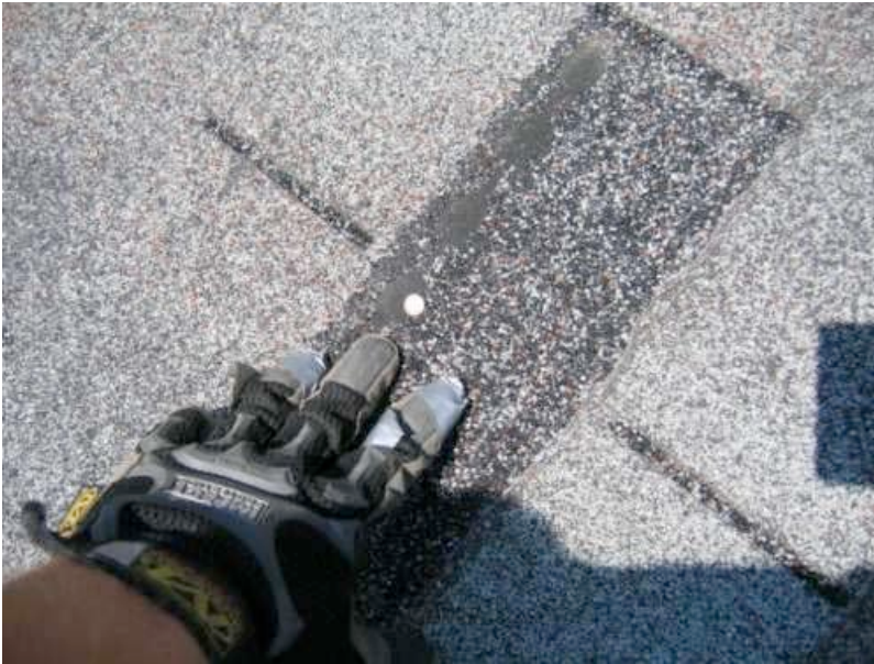
Missing shingle tab at the rear right corner of the roof. Exposed roofing nail. Prone to water penetration. Deficient.
