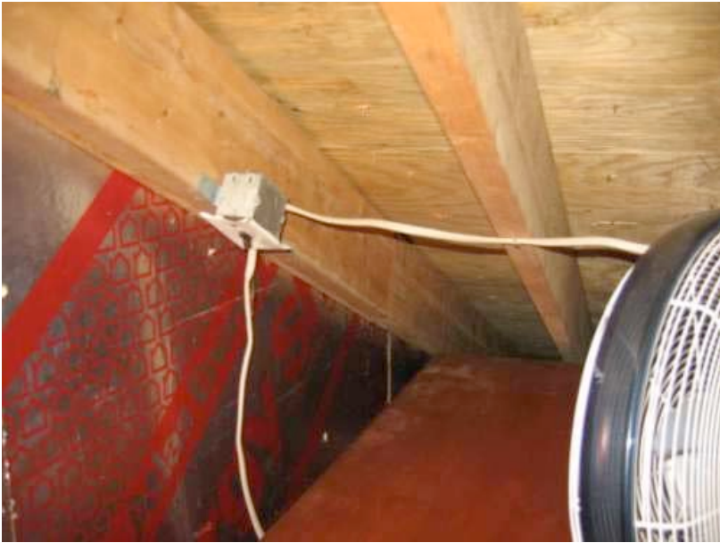
Improperly installed electrical components and wiring in the attic space. Deficient.
