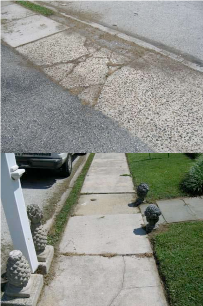
Differential movement, cracking, and uneven surfaces at the walkways.
