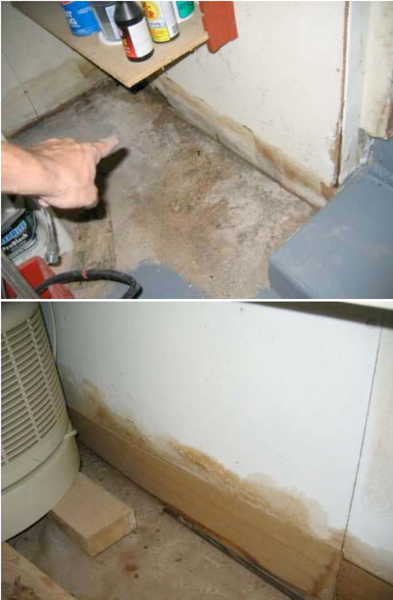
Evidence of water intrusion at the bottom of the finished walls in the basement. Deteriorated wooden materials and components at those basement walls. Deficient.
