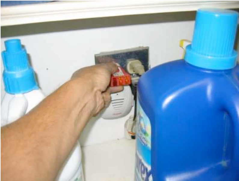
Missing GFCI protection at the laundry tub area. Deficient.
