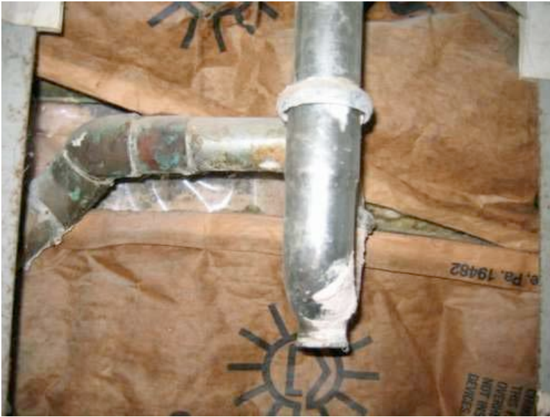
The chrome-coated soft brass drain fitting under the laundry tub is showing evidence of leaking. Deficient.
