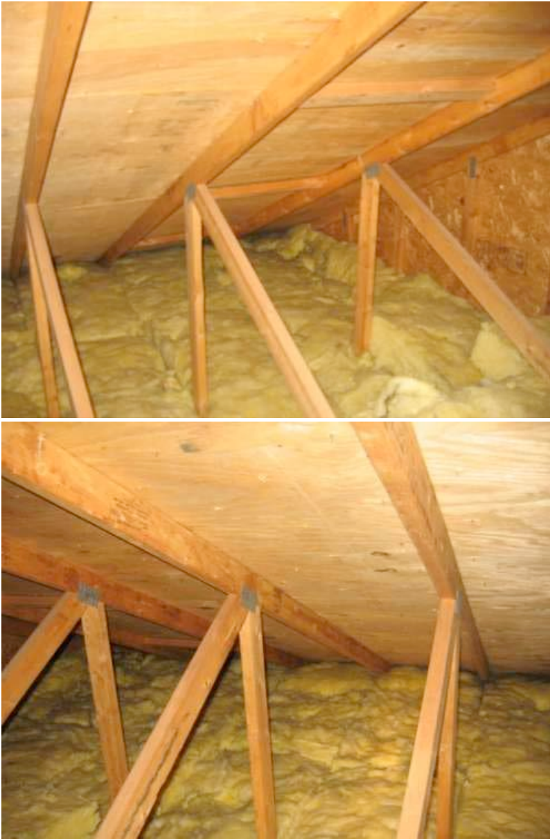
The attic space was inspected by entering it. The access was limited, because there was no flooring on which to stand or walk.
