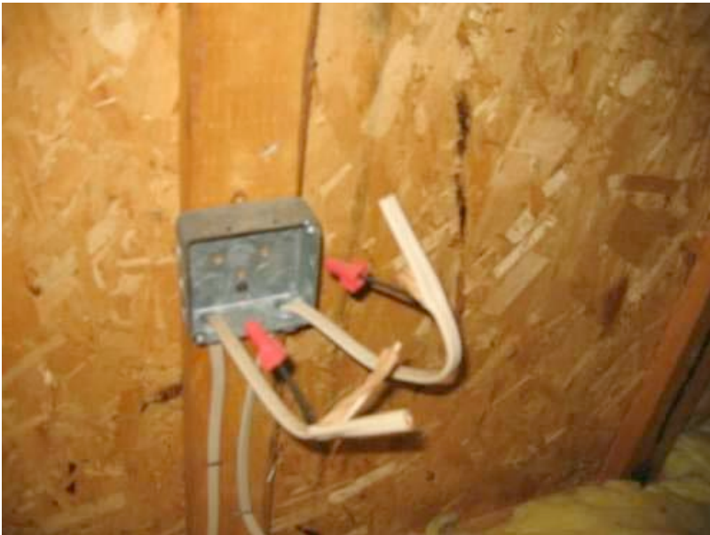
Open electrical junction box in the attic space. Deficient.
