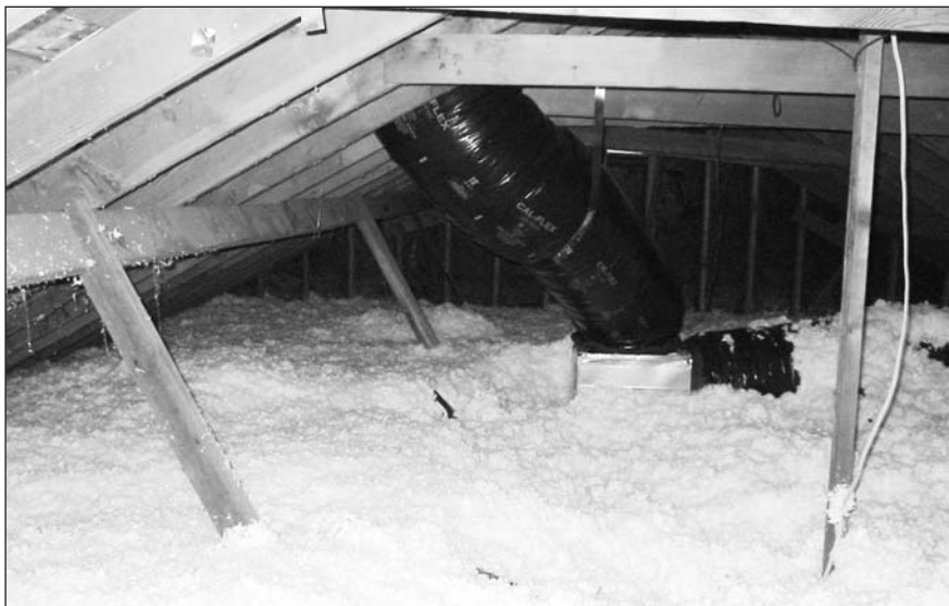
The new flex ducts in the attic are covered by additional blown-in insulation after the retrofit.
