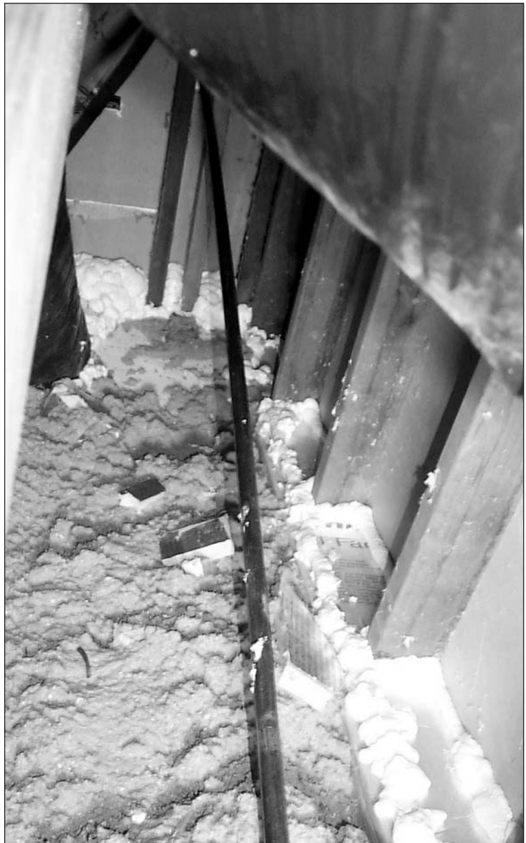
It's important to seal cavities connecting the house to the attic. Foam was used for sealing small holes and cracks at building component intersections.
