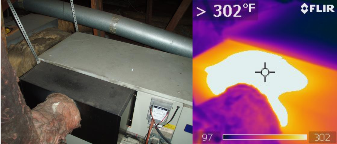
Hot spot on furnace.
