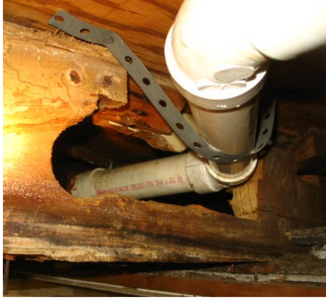
Picture of drain pipe slope and joist condition.
