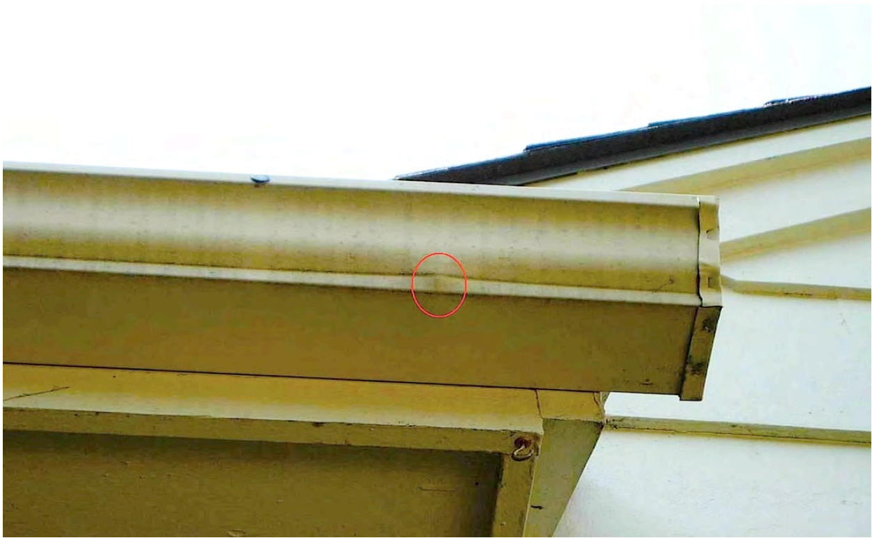
These photographs show actual hail damage to gutters.
