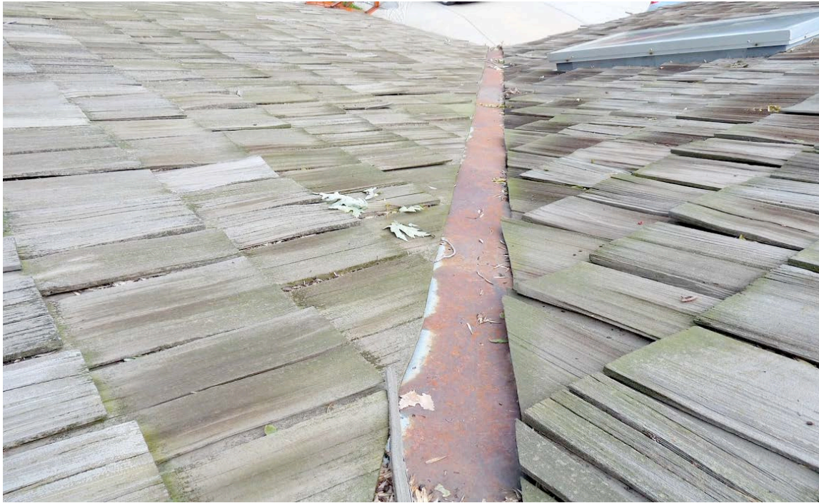
severely corroded flashing which needs replacement soon to avoid damage from moisture intrusion
